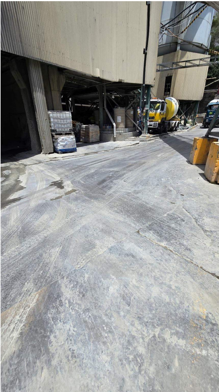
Figure 43 Cracks observed (40, 41, 42, 43, 44) - Concrete cracks throughout area
