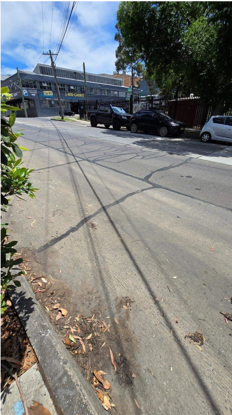
Figure 39 Cracks observed (37, 38, 39) - Road exhibits substantial joint sealant repairs, several cracks observed throughout road
