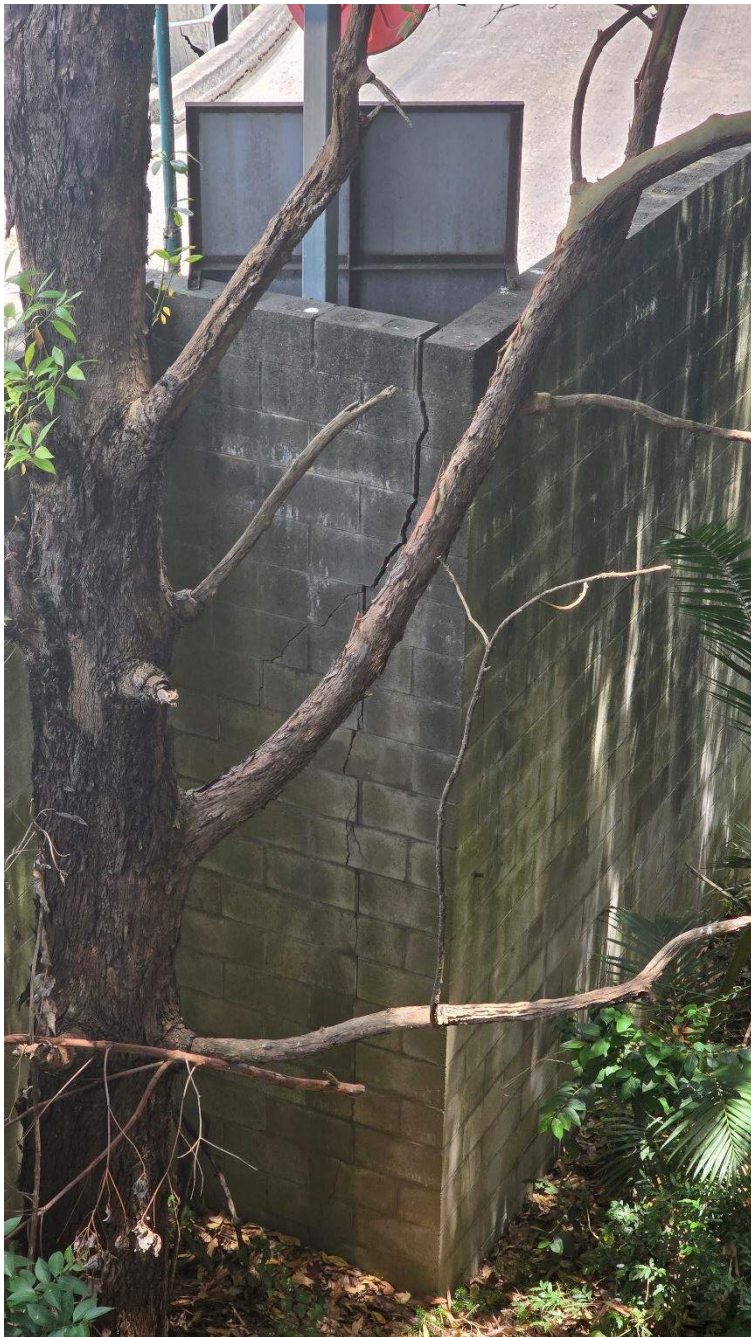
Figure 45 Cracks observed (45) - Retaining wall large vertical crack
