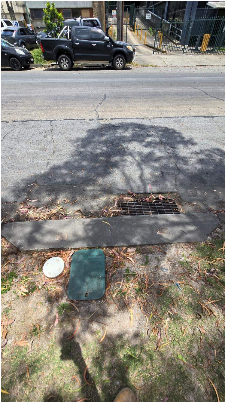
Figure 10 Cracks observed (9, 10) - Large surface breaks footpath
