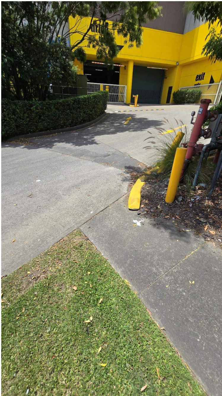
Figure 7 Cracks observed (7) - Large surface breaks driveway
