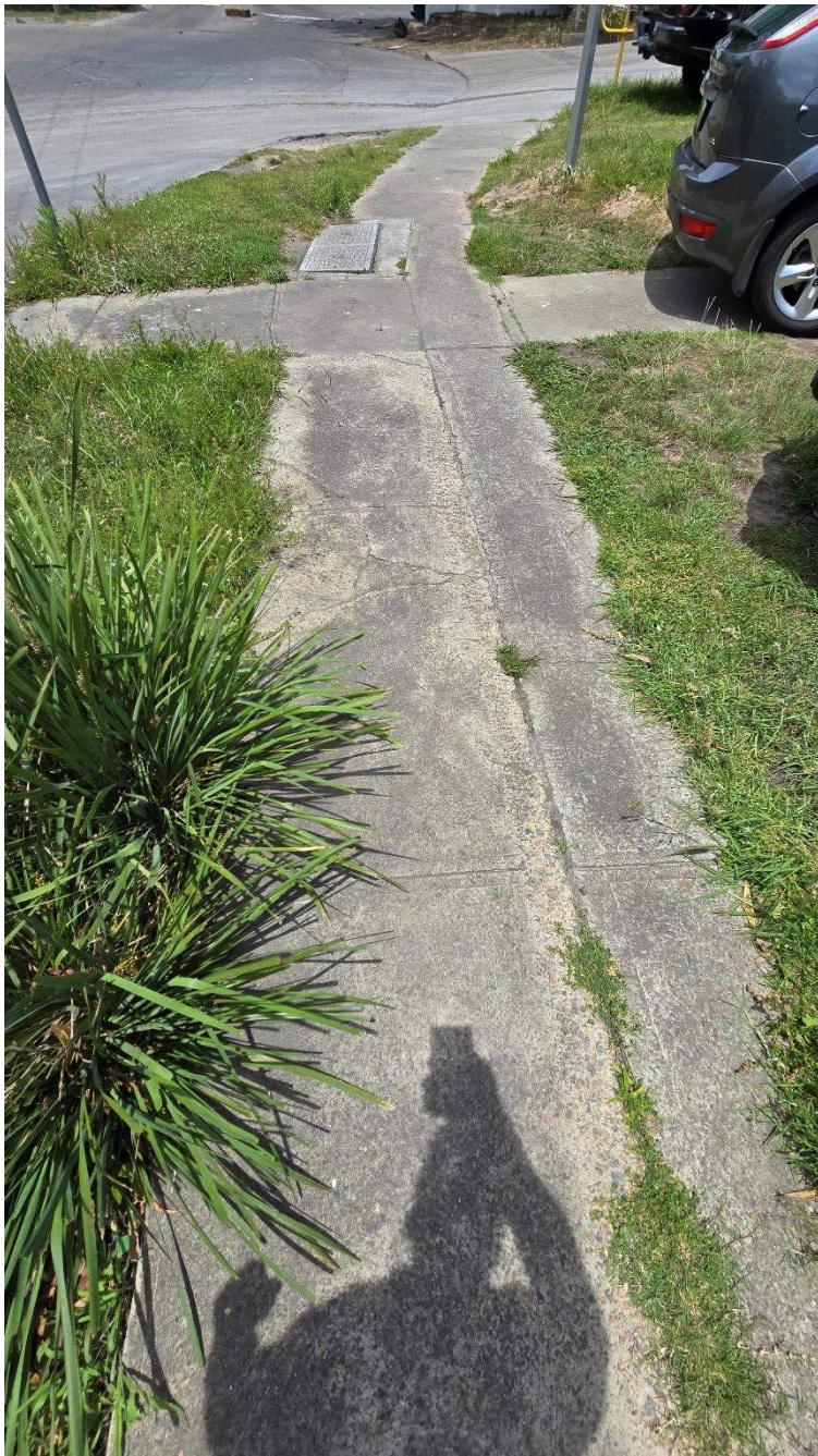
Figure 2 Cracks observed (2) - Tree root infestation in footpath
