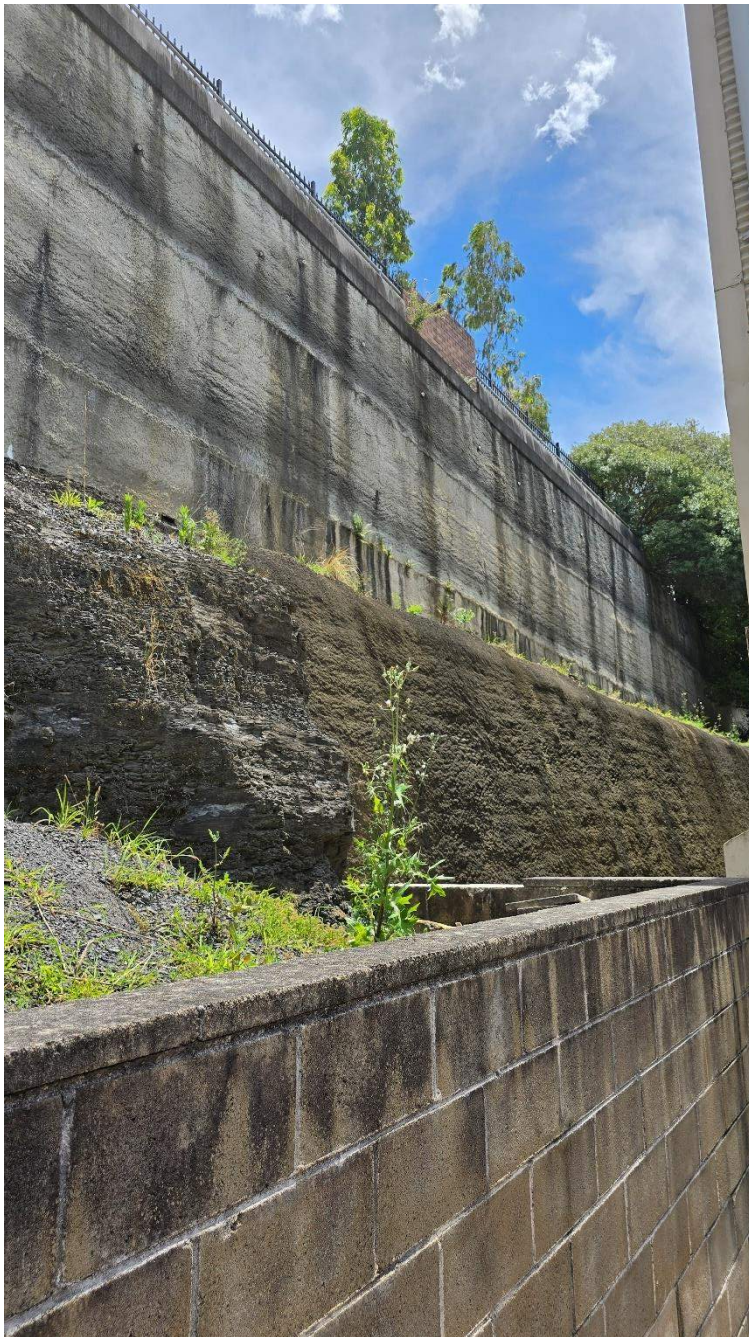
Figure 48 Cracks observed (46, 47, 48, 49) - Retaining wall exhibited signs of horizontal surface cracking
