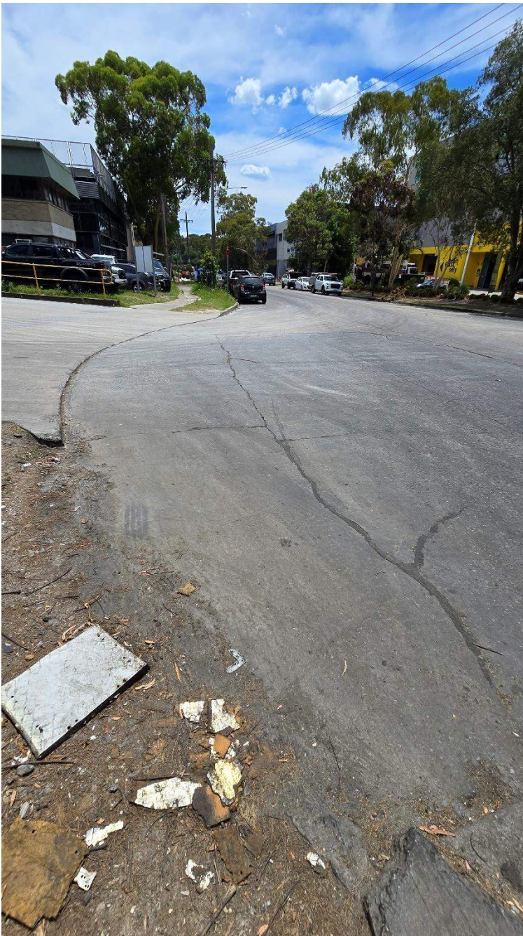
Figure 5 Cracks observed (5) - General wear and tear of driveway
