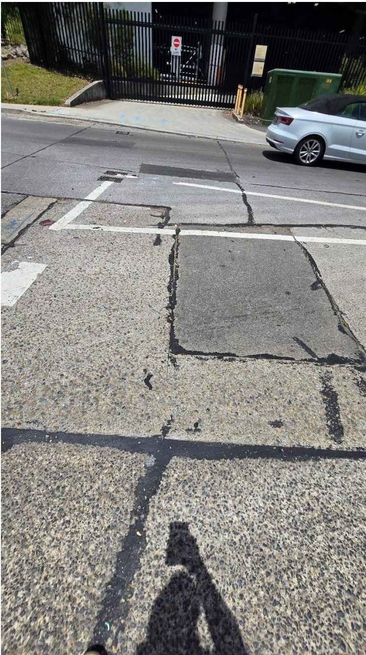
Figure 35 Cracks observed (34, 35) - Road exhibits substantial joint sealant repairs, several cracks observed throughout road
