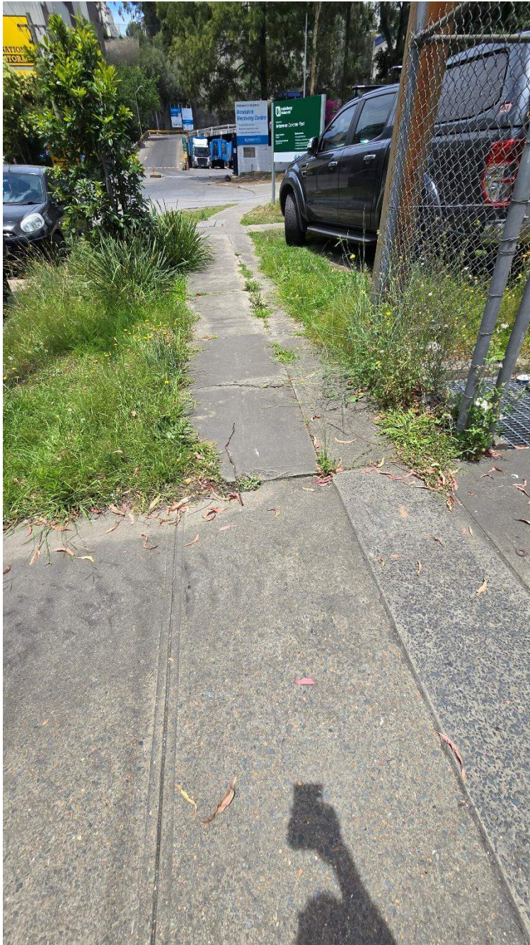
Figure 1 Cracks observed (1) - Crocodile cracking developing
