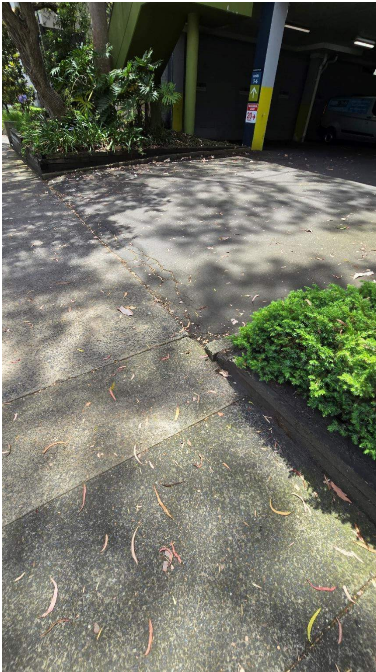
Figure 20 Cracks observed (21) - Crocodile cracking in driveway
