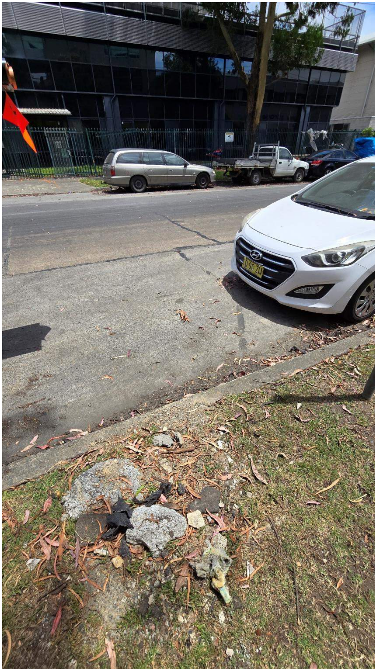
Figure 12 Cracks observed (12, 13, 14) - Large surface breaks road
