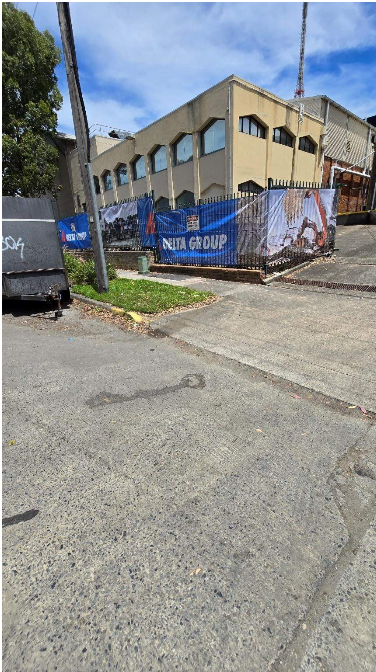
Figure 26 Cracks observed (25, 26, 27) - Road in poor condition, cracks and repairs observed throughout
