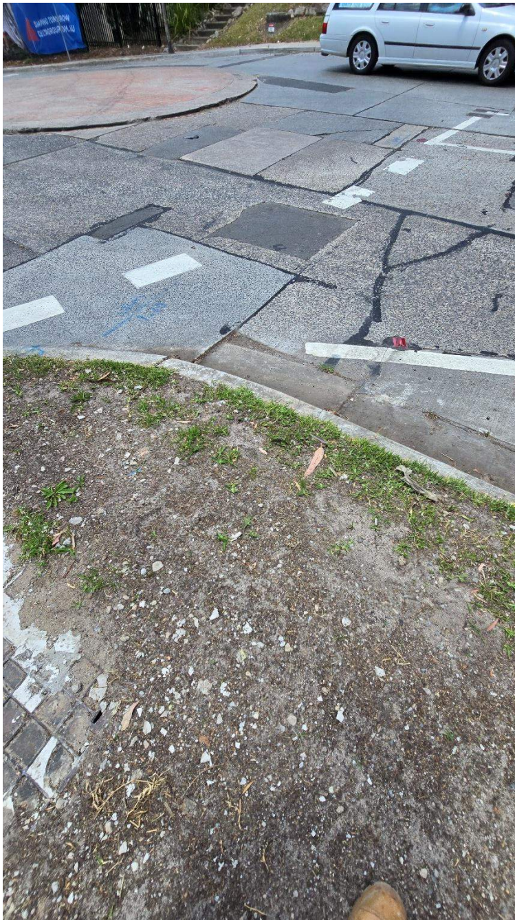
Figure 34 Cracks observed (34, 35) - Road exhibits substantial joint sealant repairs, several cracks observed throughout road
