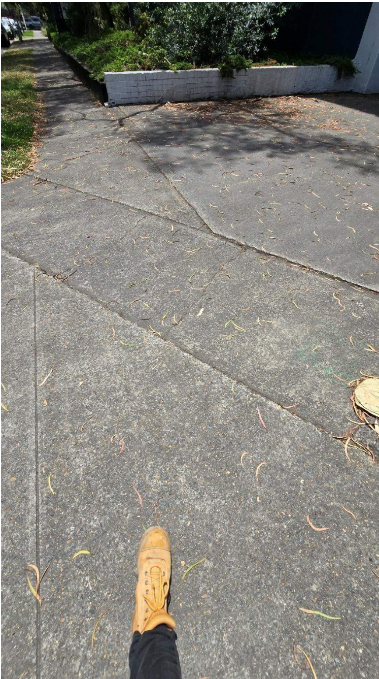
Figure 18 Cracks observed (19) - Poor condition of driveway, cracks and joints
