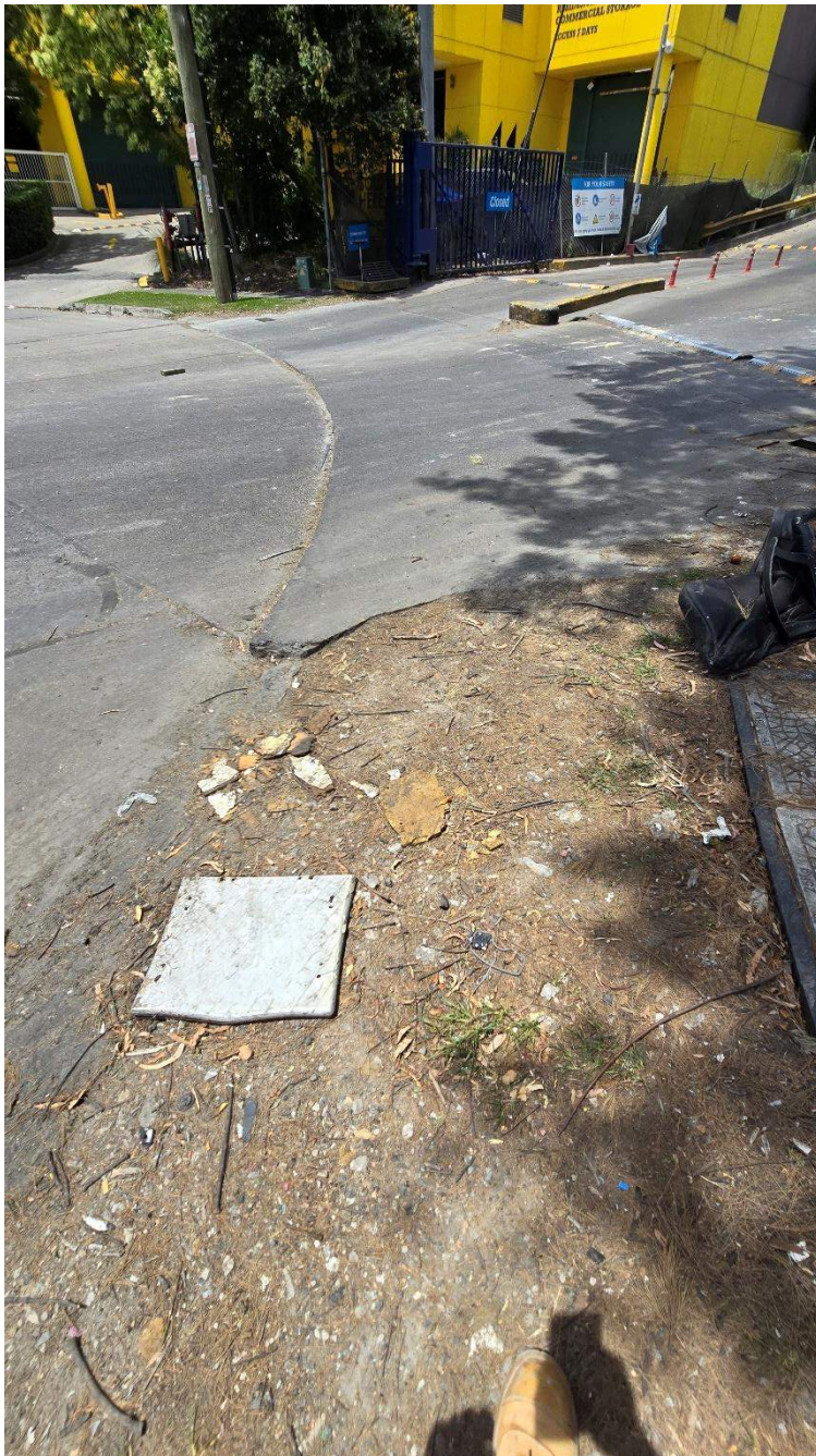
Figure 4 Cracks observed (4) - Crocodile cracking developing
