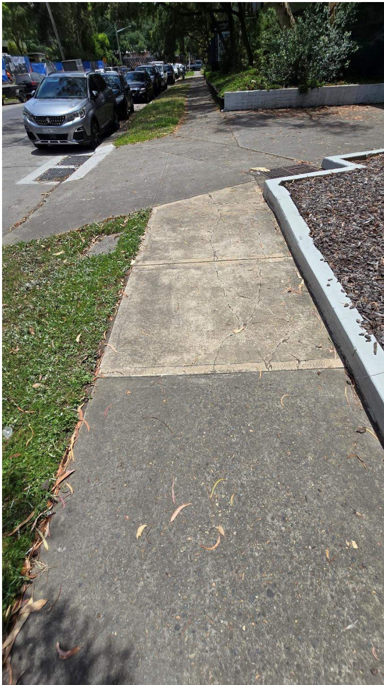
Figure 17 Cracks observed (18) - Footpath concrete cracks
