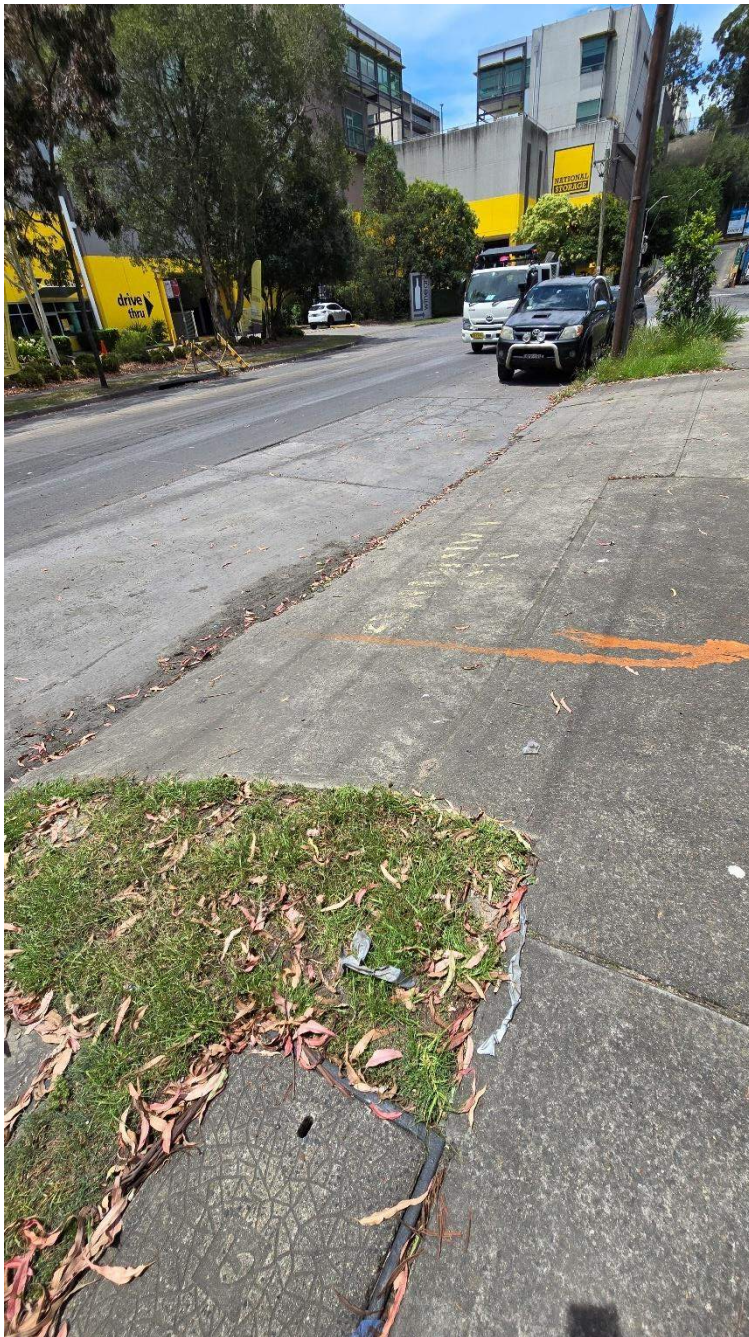
Figure 30 Cracks observed (28, 29, 30) - Footpath cracking
