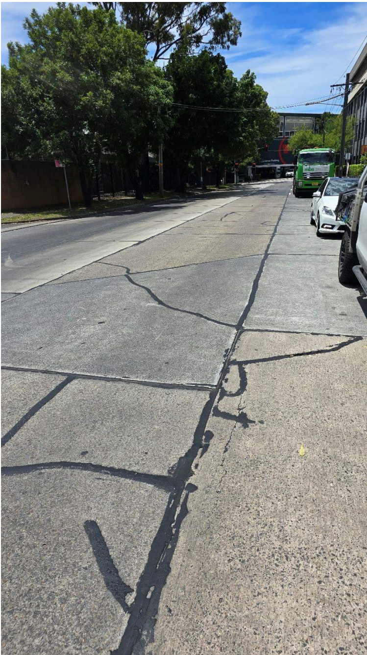
Figure 33 Cracks observed (32, 33) - Road exhibits substantial joint sealant repairs, several cracks observed throughout road
