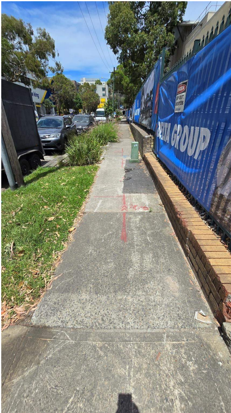
Figure 27 Cracks observed (28, 29, 30) - Footpath cracking
