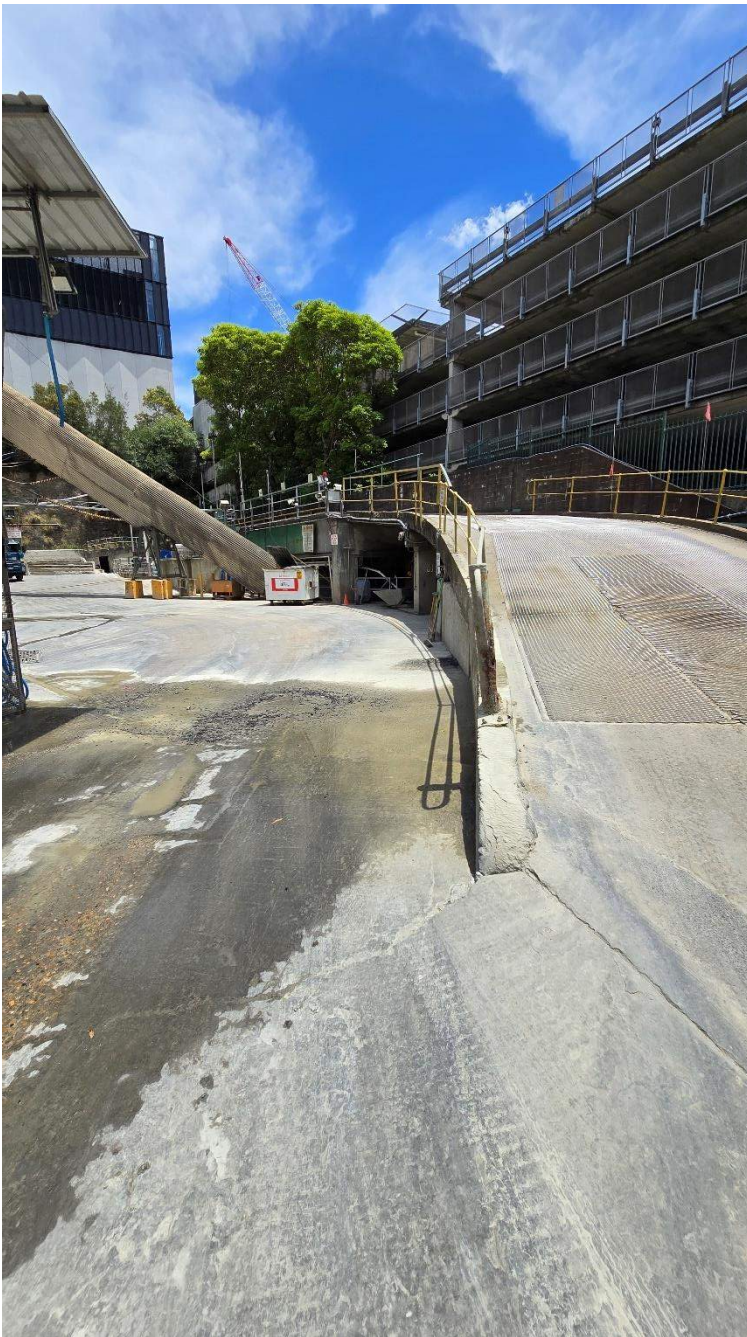
Figure 40 Cracks observed (40, 41, 42, 43, 44) - Concrete cracks throughout area
