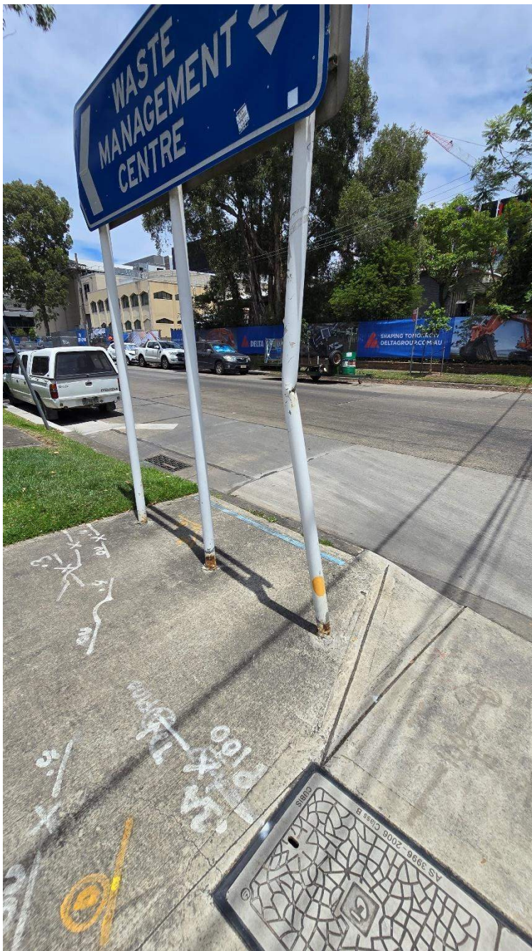
Figure 31 Cracks observed (31) - Sign has been struck and deformed
