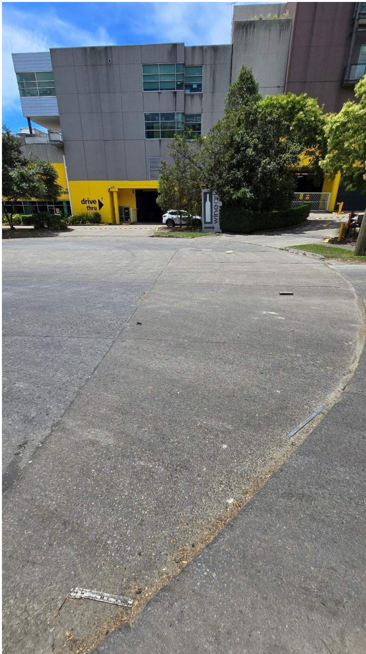
Figure 6 Cracks observed (6) - Large surface breaks road
