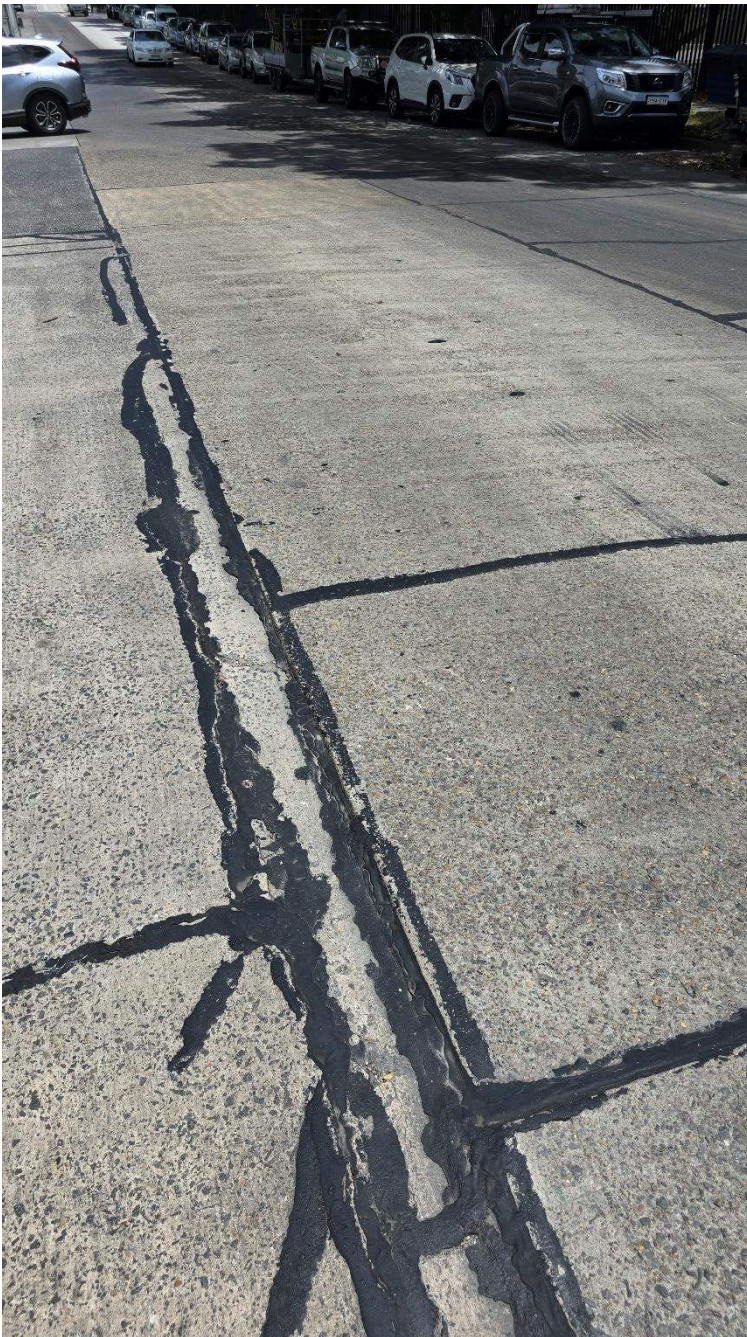
Figure 32 Cracks observed (32, 33) - Road exhibits substantial joint sealant repairs, several cracks observed throughout road
