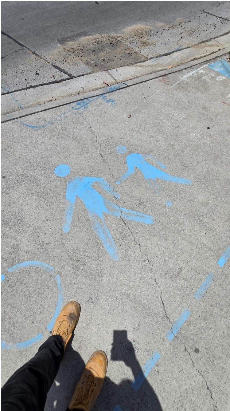
Figure 36racks observed (36) - Surface breaks driveway
