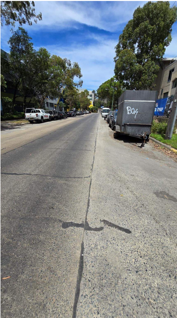
Figure 25 Cracks observed (25, 26, 27) - Road in poor condition, cracks and repairs observed throughout
