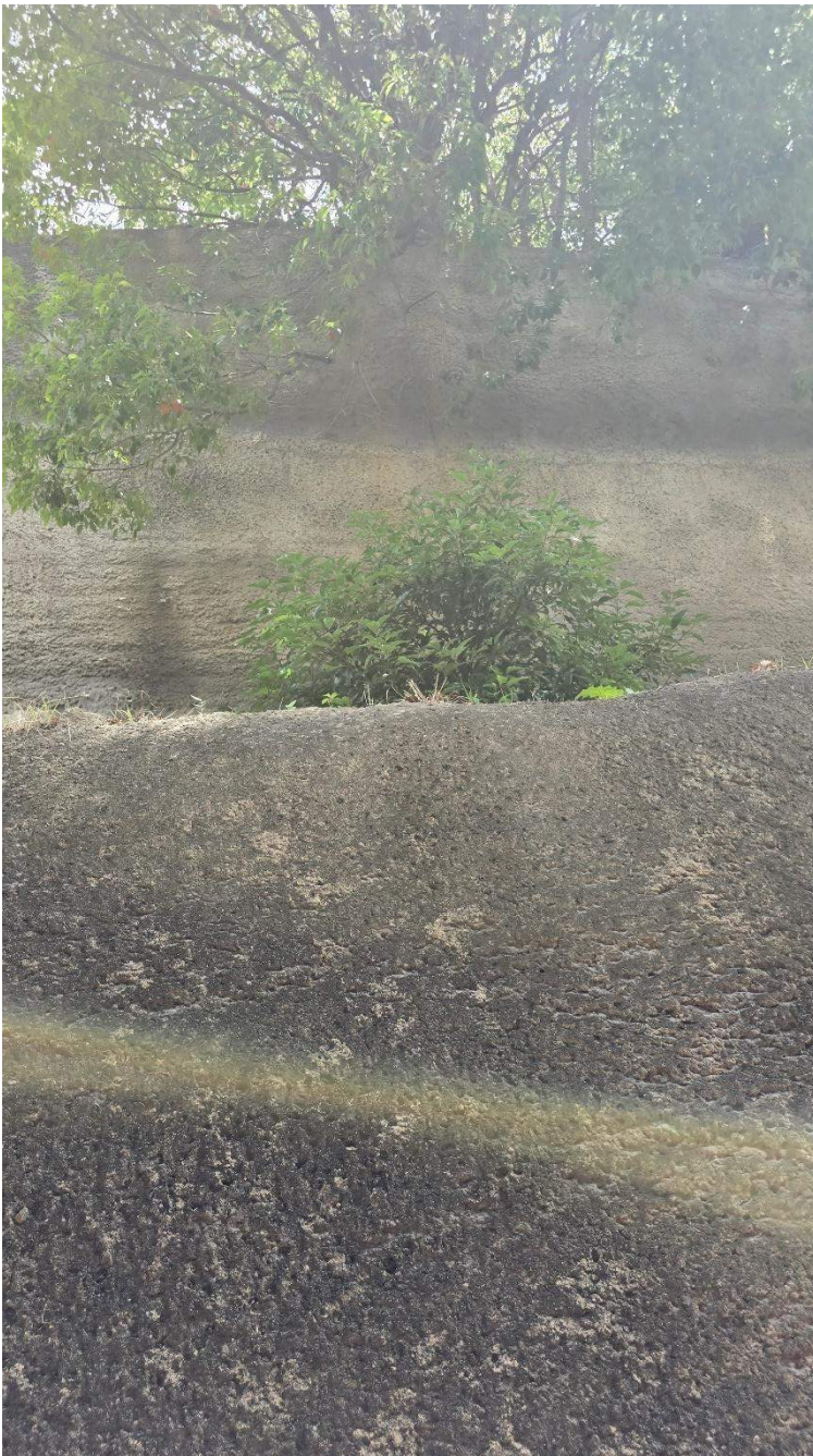
Figure 49 Cracks observed (46, 47, 48, 49) - Retaining wall exhibited signs of horizontal surface cracking
