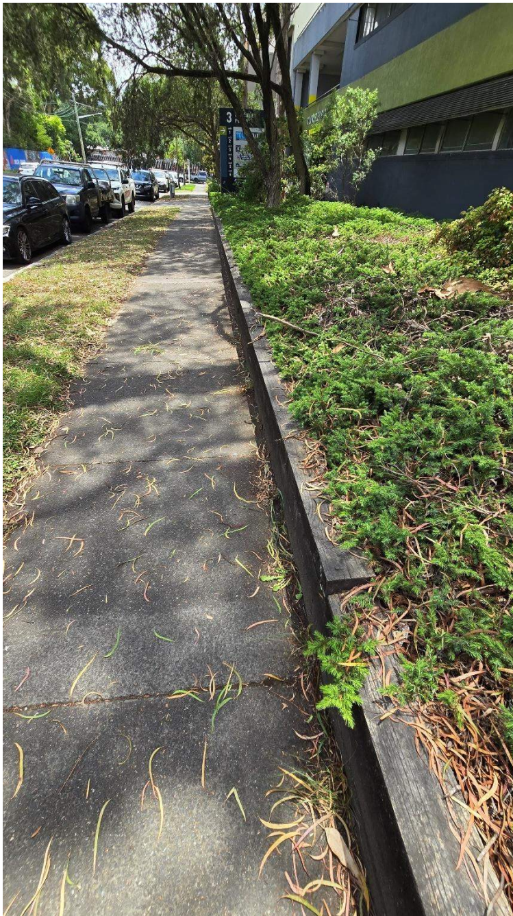
Figure 19 Cracks observed (20) - Retaining wall leaning outwards
