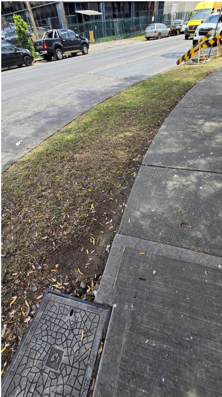
Figure 9 Cracks observed (9, 10) - Large surface breaks footpath
