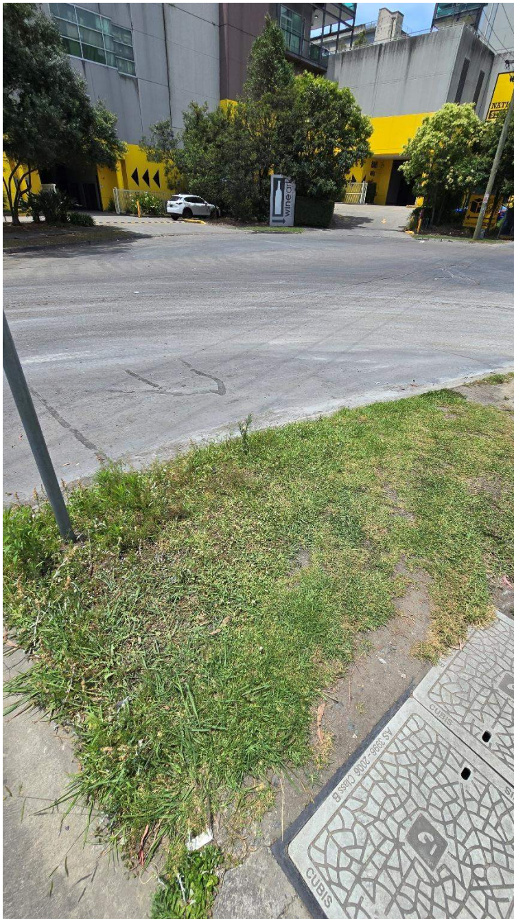
Figure 3 Cracks observed (3) - Substantial cracking in pavement
