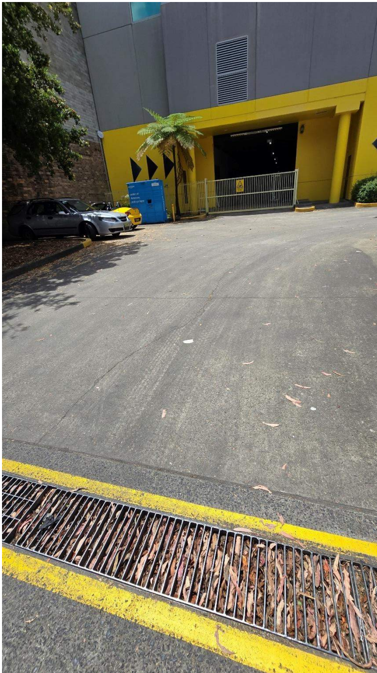
Figure 14 Cracks observed (15) - Large surface breaks driveway
