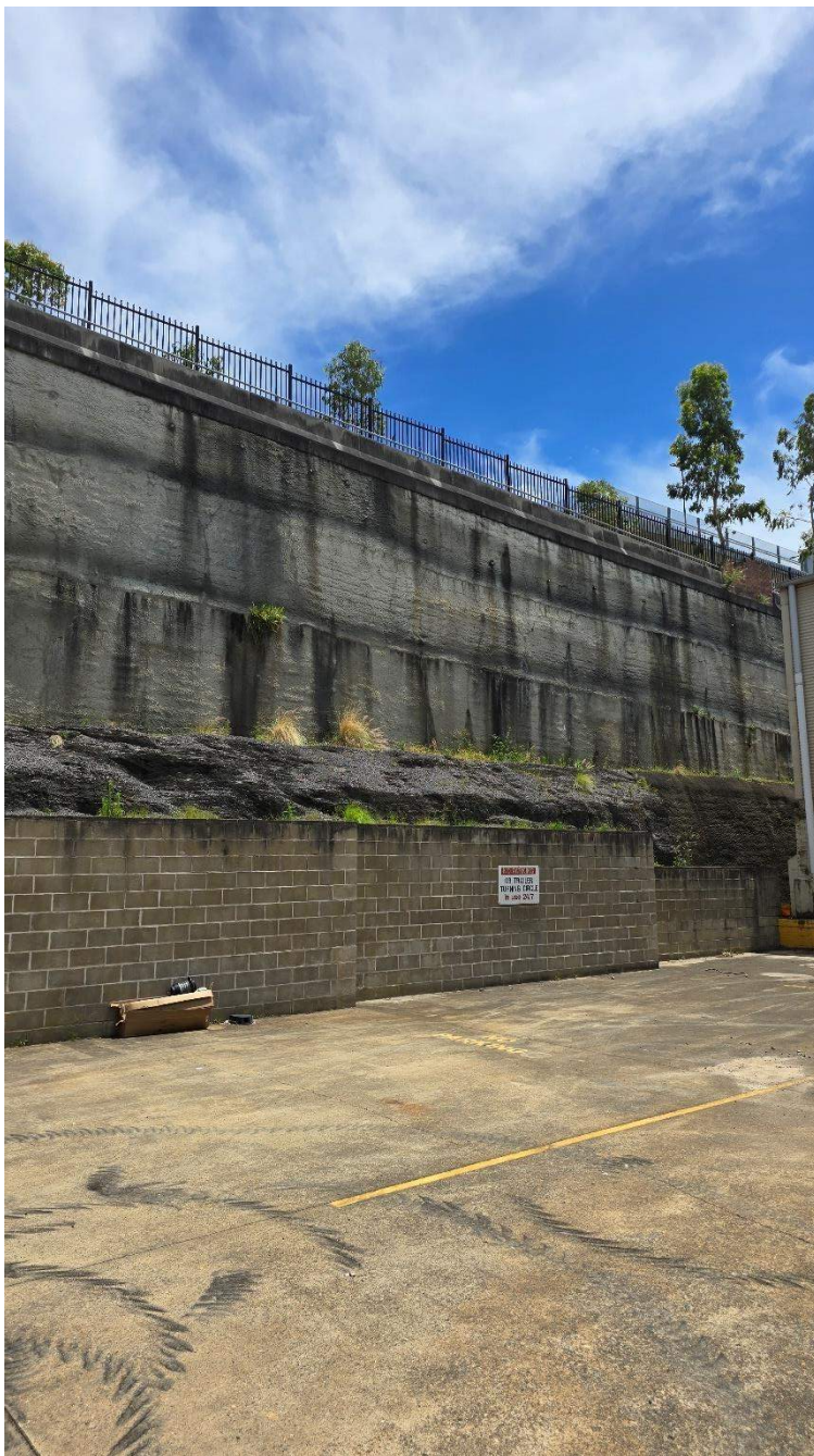
Figure 47 Cracks observed (46, 47, 48, 49) - Retaining wall exhibited signs of horizontal surface cracking
