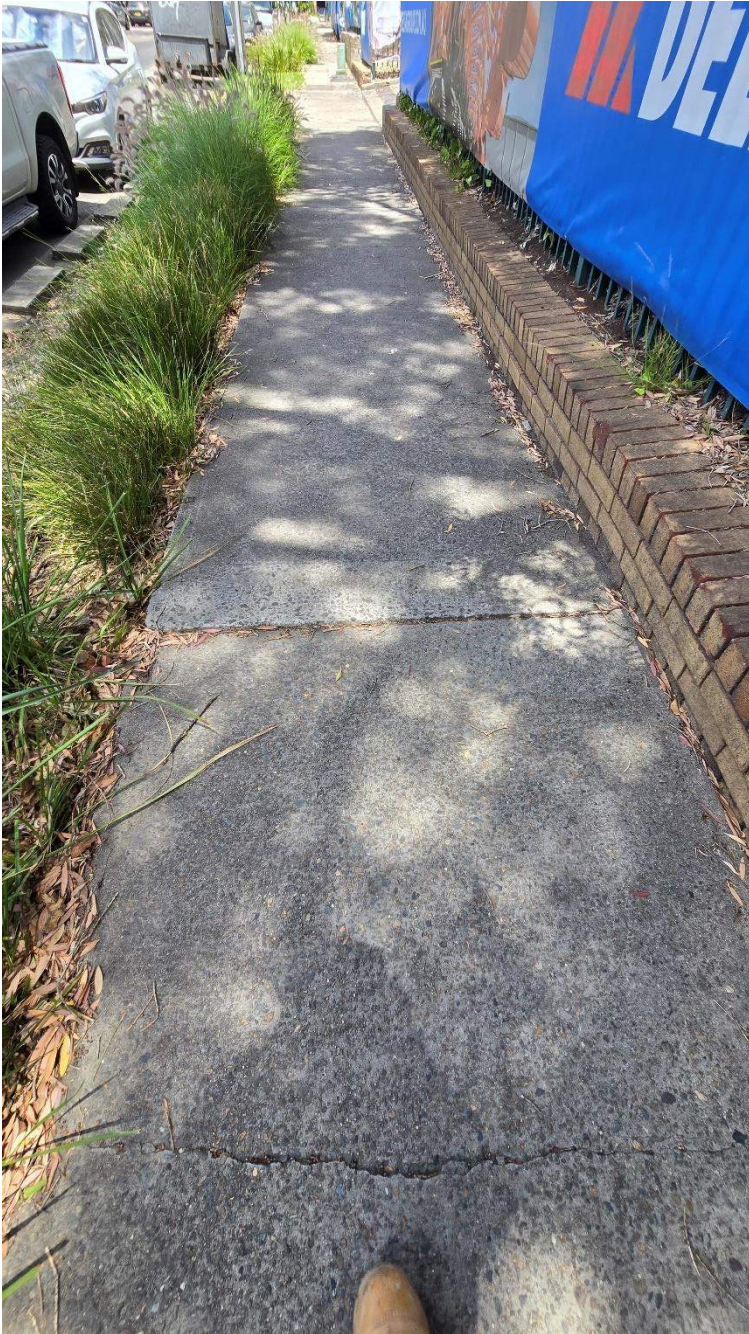
Figure 23 Cracks observed (24) - Footpath cracking
