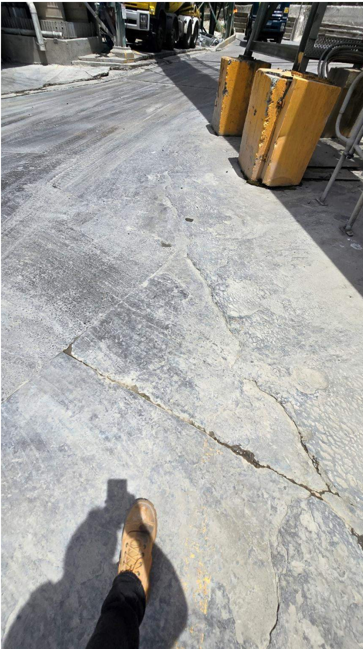
Figure 44 Cracks observed (40, 41, 42, 43, 44) - Concrete cracks throughout area
