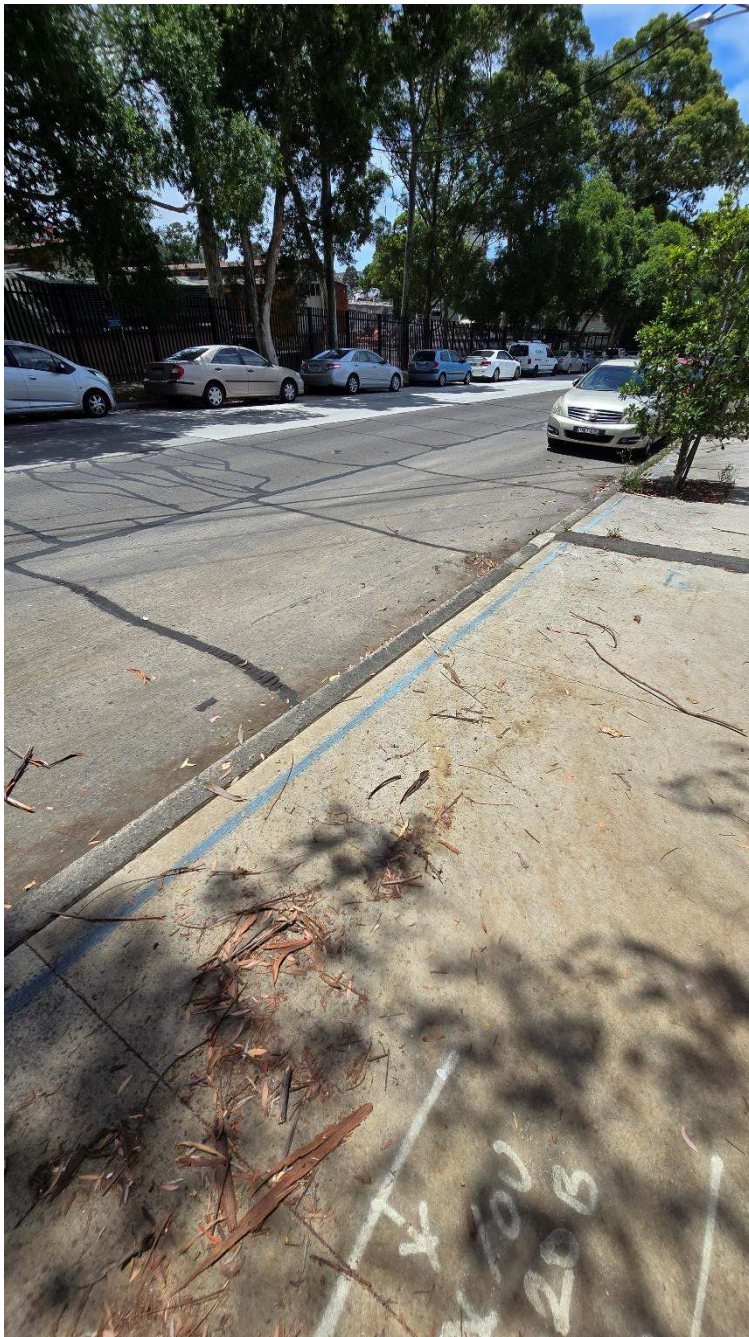
Figure 38 Cracks observed (37, 38, 39) - Road exhibits substantial joint sealant repairs, several cracks observed throughout road
