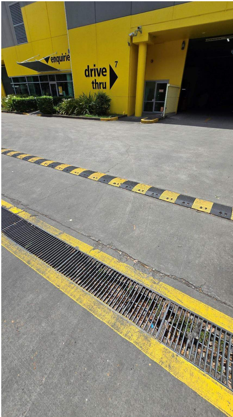
Figure 8 Cracks observed (8) - Large surface breaks driveway
